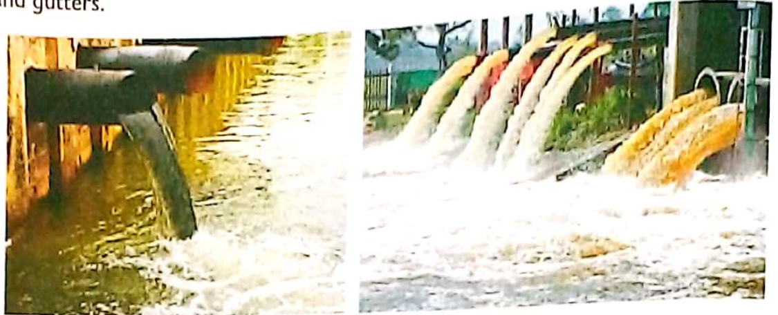
Sewers or sewage pipes connected into water bodies
